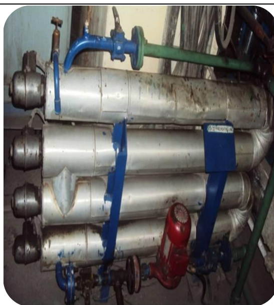
Figure 7.7 Electrical Heating System
