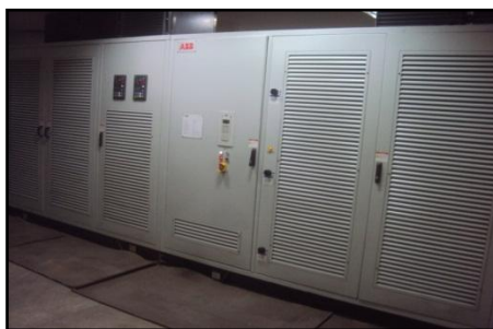
Figure 7.9 VFD for Line-2 Cement Mill bag filter fan
