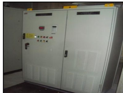
Figure 7.10 VFD Line-2 Pre-heater ID Fan
